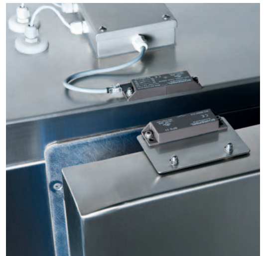
Electrical safety detection systems
