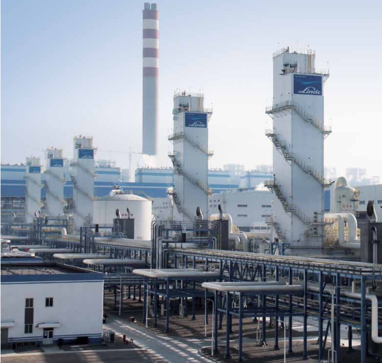
Air separation units near Yinchuan, China.
