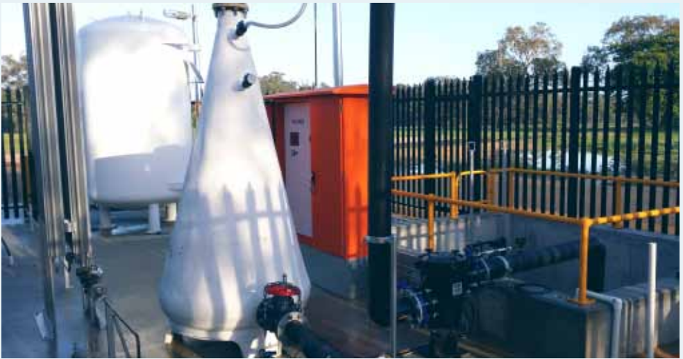
SOLVOX C-110 installation at one of the four oxygenation plants on the Canning and Swan rivers.
