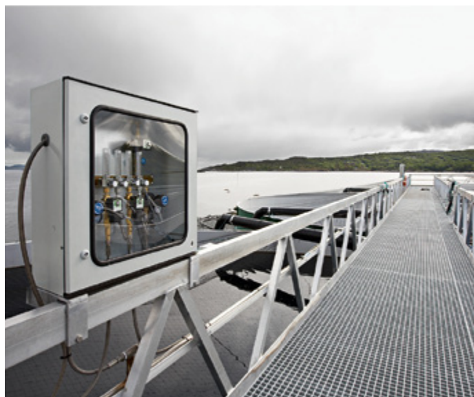
Control cabinet installation on a fish farm site.
